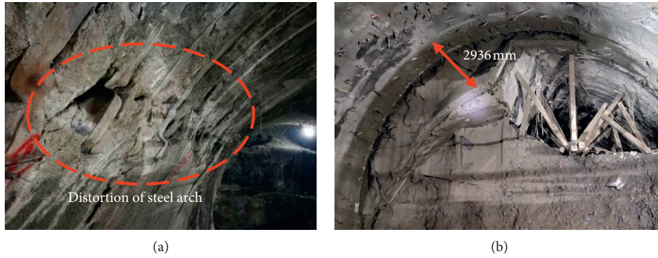
FIGURE 5: Deformation and failure characteristics of primary lining. (a) Distortion of steel arch. (b) Large deformation of the surrounding rock.
